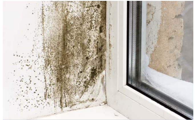
Condensation mould is unsightly and can cause health problems
